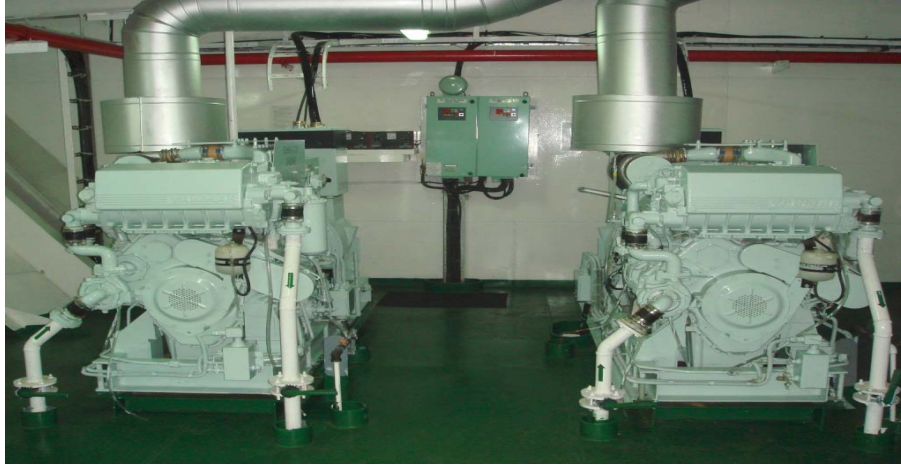
Engine Room – Auxiliary Engines
