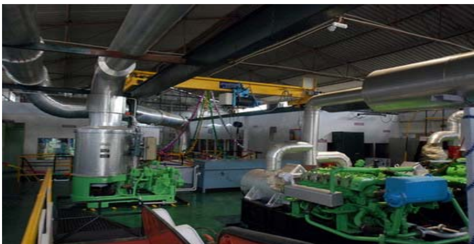
Engine Room – Machineries
