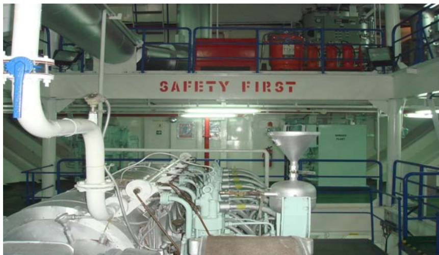
Engine Room – Main Engine
